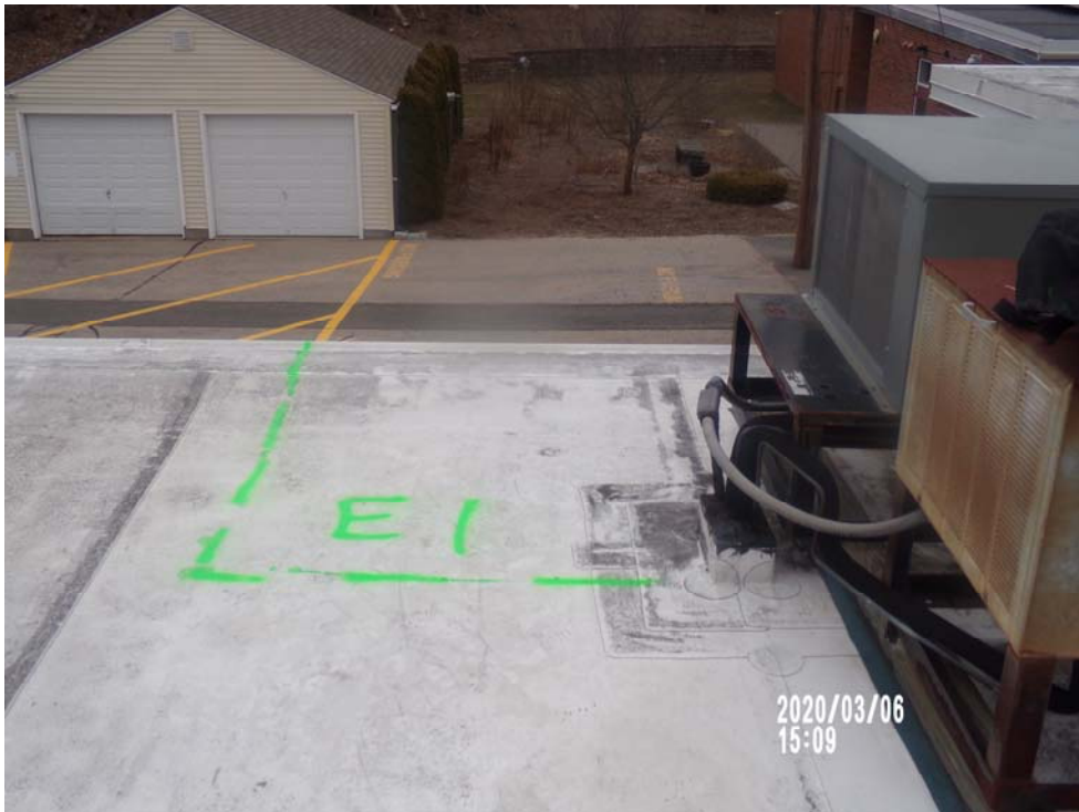
Roof E-Suspected wet area E-1, West side, looking North
