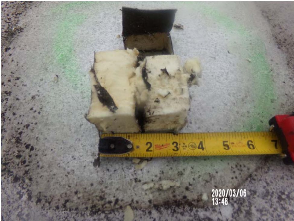
Roof A-Core cut #CC2 at wet area #A1 (Wet)
