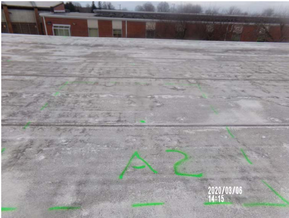
Roof A-Suspected wet area A-2, looking South
