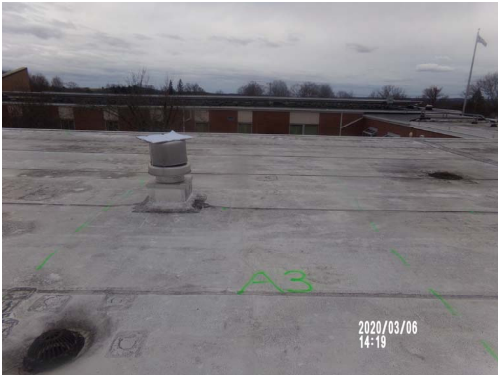
Roof A-Suspected wet area A-3, center, looking South
