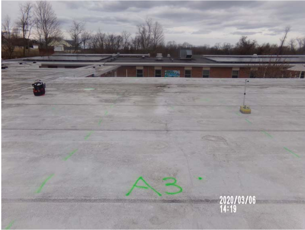
Roof A-Suspected wet area A-3, center, looking North
