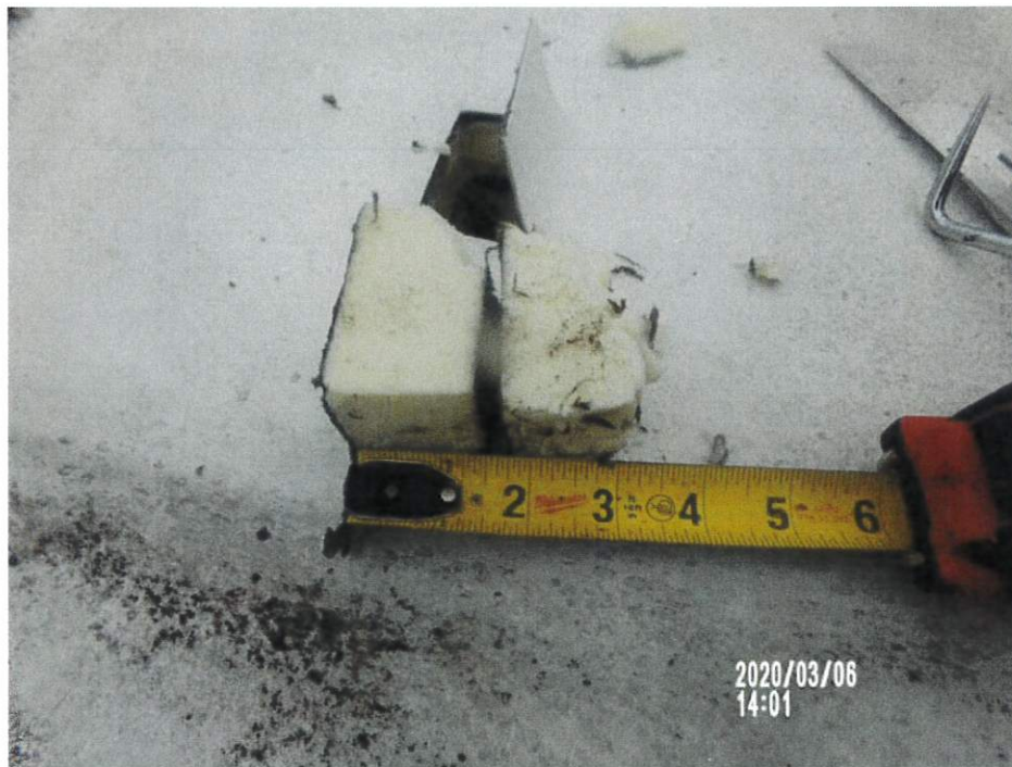
Roof A-Core cut #CC3 at wet area #A1 (Wet)
