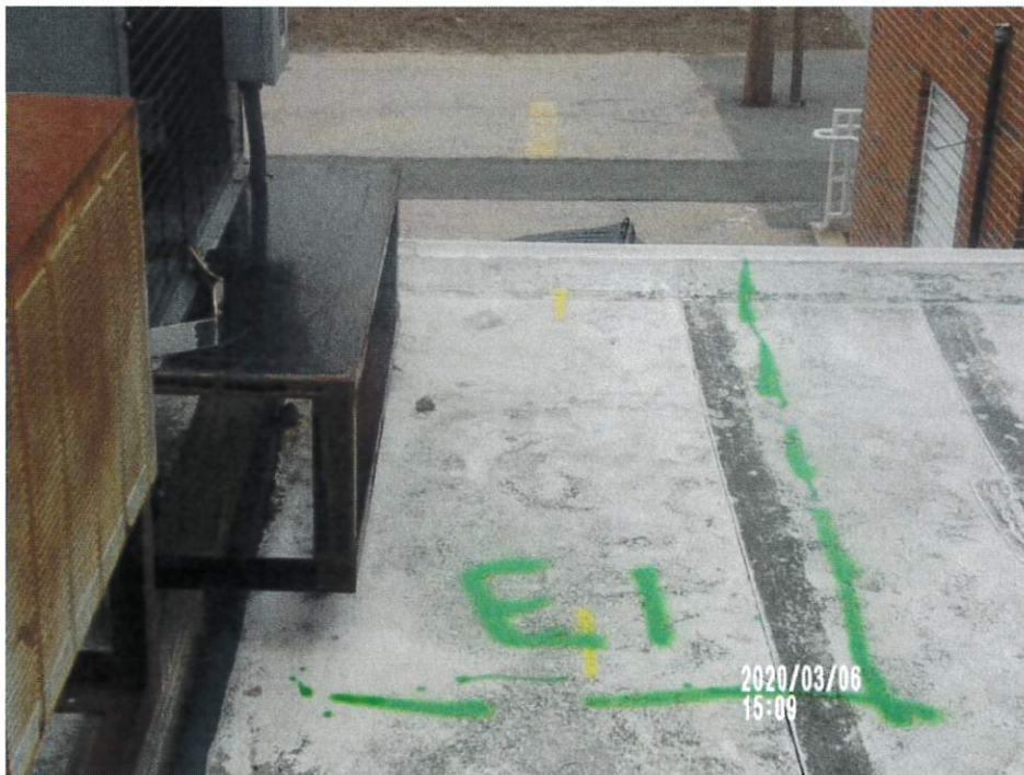
Roof E-Suspected wet area E-1, East side, looking North
