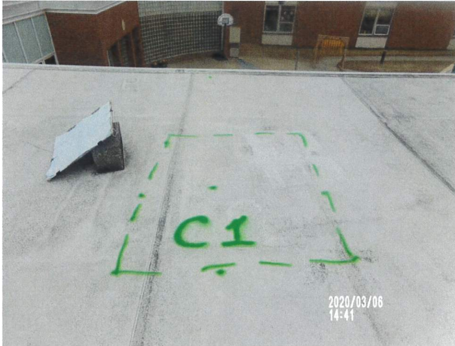
Roof C-Suspected wet area C-1, looking South
