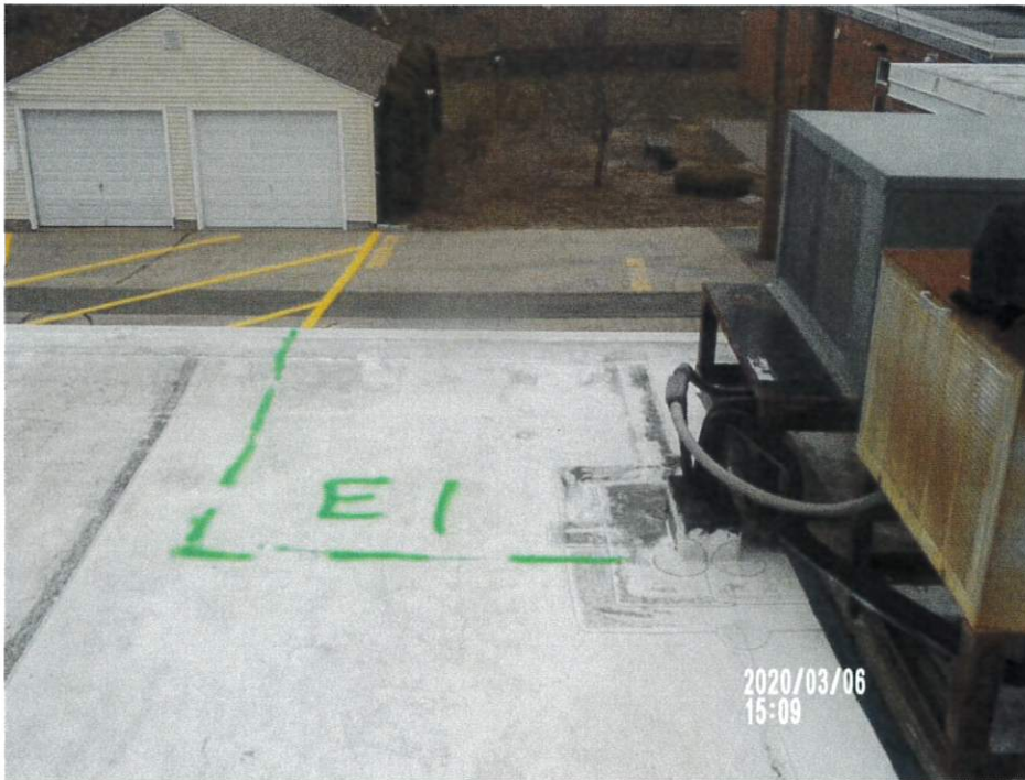
Roof E-Suspected wet area E-1, West side, looking North
