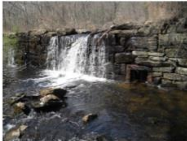
Dam at Hodge's Mill as it appears in 2016. Photo taken on the east side of the river looking westerly.
